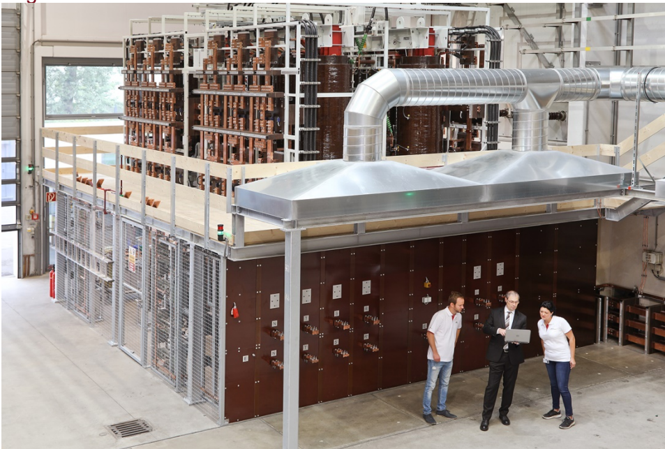
Image caption: At the heart of the DC lab is the switchgear, consisting of two parts: four transformers at the top level, and rectifiers which convert alternating current to direct current at the bottom level. Both levels are designed for very high currents of up to 80 kA and 75 MW test performance. © AIT/Krischanz
